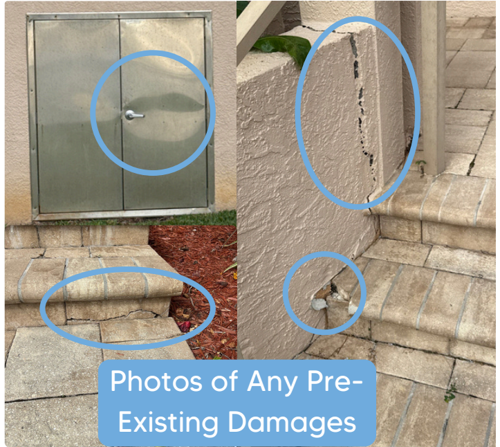
Document Driveway cracks
